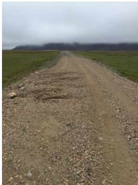
Photo No. 12 – 14 August 2016; 1245 hours. Washout near Suqi River culvert. View facing southeast.
