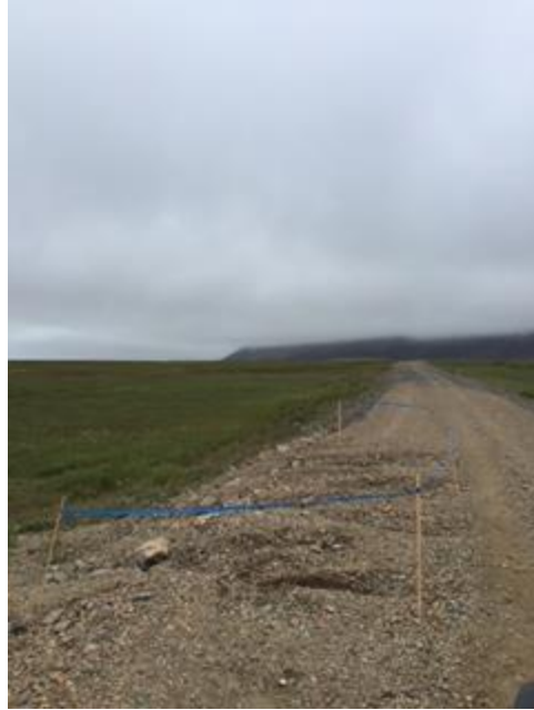
Photo No. 13 – 14 August 2016; 1253 hours. Flagging placed as safety barrier around washout near Suqi River culvert. View facing southeast.
