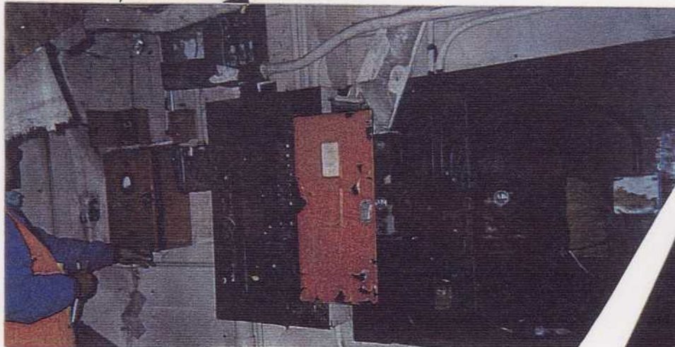
EAST WALL GROUP WASTINGHOUSE PANEL BOX- 15 BREAKERS
