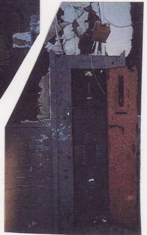
WEST WALL SWITCH BOX
