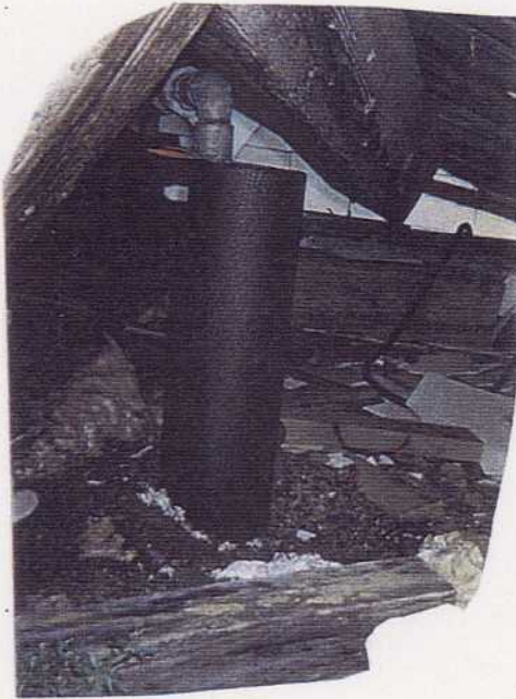
↑ WELL #1, SOUTH OF BLDG. 113
